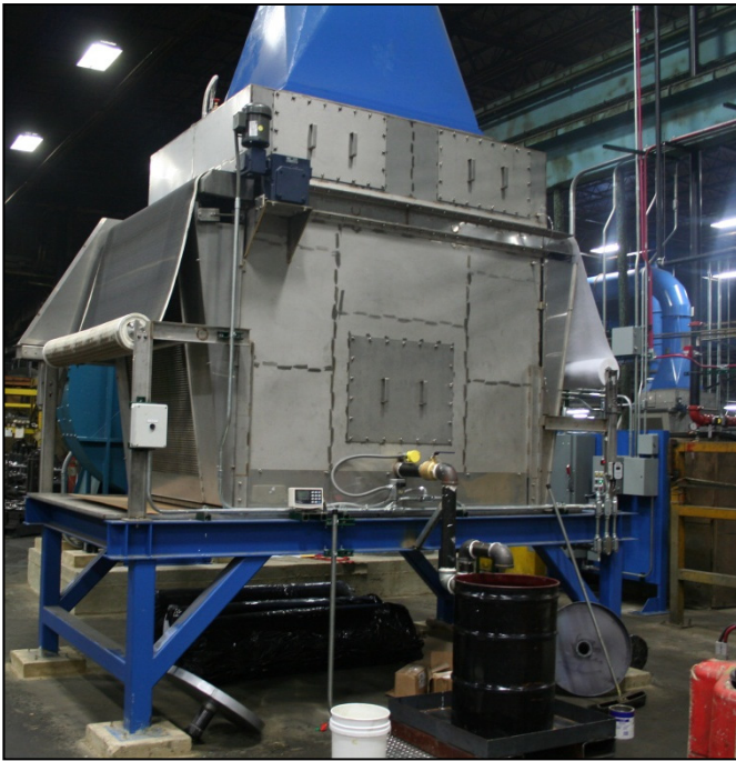
UHF® installation at a metal products plant.
